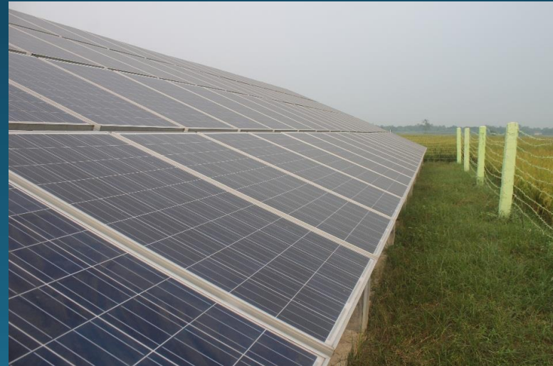
Solar PV installed for irrigation pump
