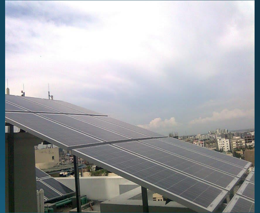
Roof Top Solution
