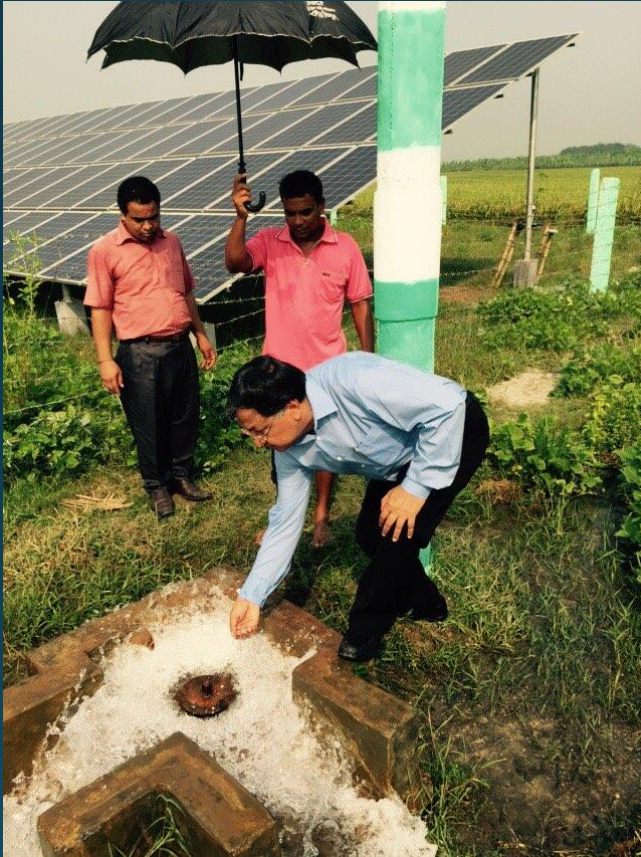
Water Discharge by a Solar Irrigation Pump installed by BGEF
